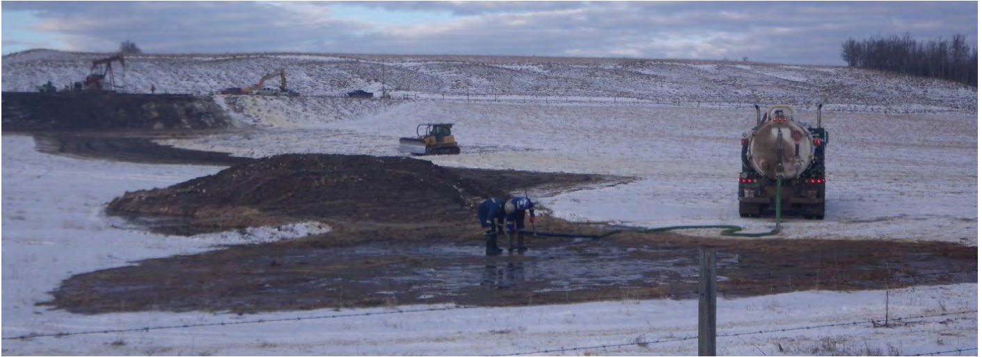
Workers stand in secret frack fluids after a frack communication blowout, Innisfail, Alberta. Photo - Alberta Surface Rights Group
