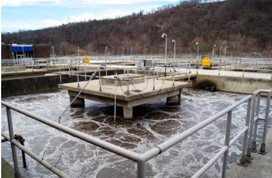
The McKeesport Sewage Treatment Plant, one of nine plants on the Monongahela River that has treated wastewater from Marcellus Shale drilling operations. (Joaquin Sapien/ProPublica)
